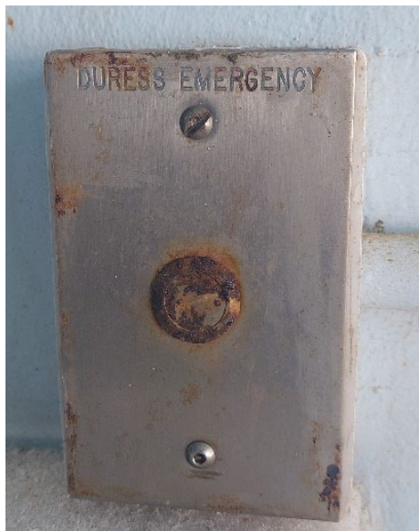
Image 1: Duress alarm in exercise yard
